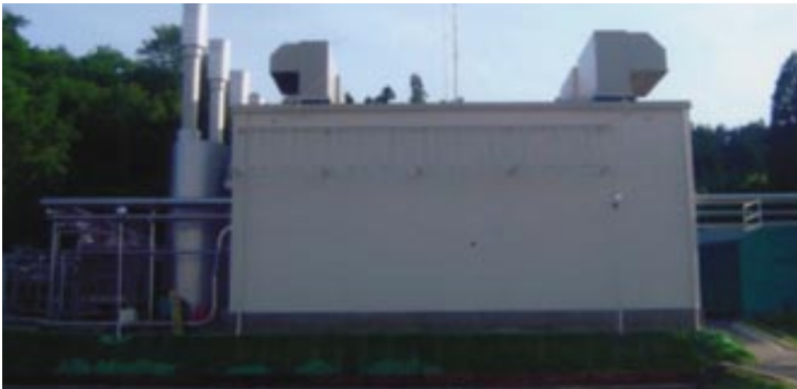
Cogeneration system unit
