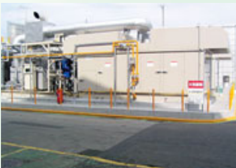
Cogeneration system introduced in the Kakogawa factory
