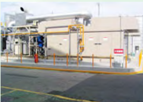
Cogeneration system introduced in the Kakogawa factory
