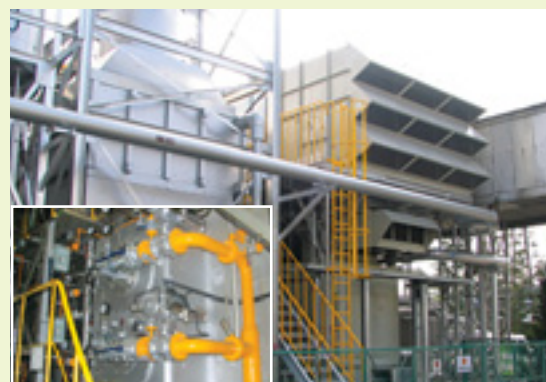
A cogeneration system is installed at the Nagoya factory.
