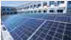
Rooftop solar panels
