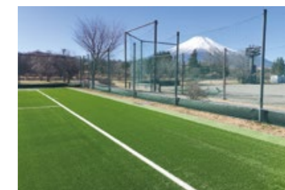
Installation of a system for curbing microplastic dispersion
